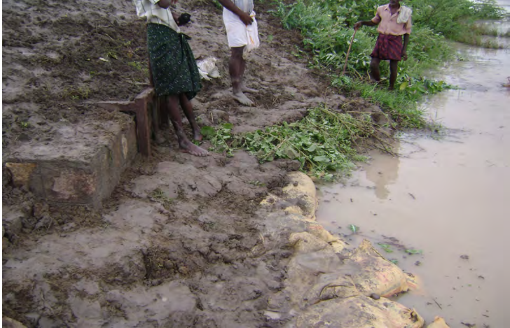
MELMANDAI TANK –DAMAGED SLUICE
